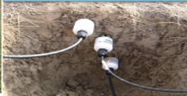
Typical soil sensor installation
